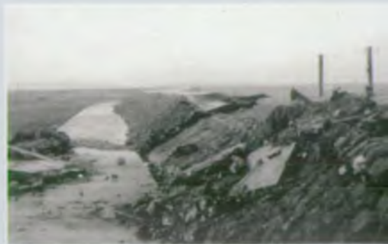
Damage to the western end of Clevedon sea wall following the storm of December 1981
