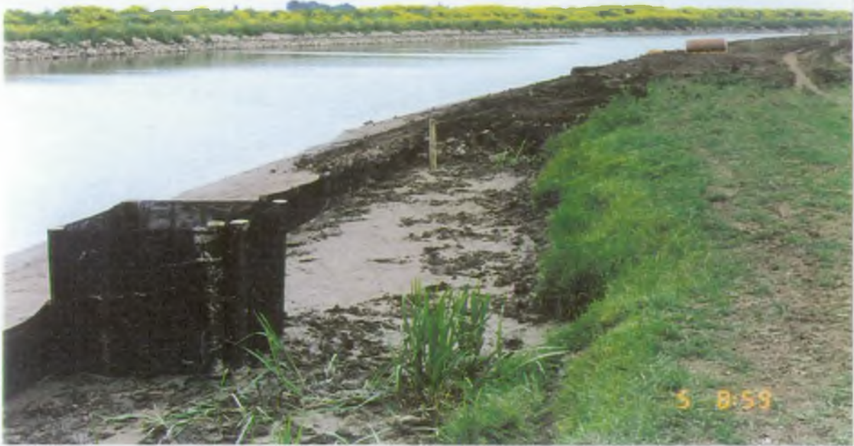
Figure. 7b : Four Mile Bar Erosion Protection, Incorporating Fishing Platforms Showing Nicospan Prior To Backfilling
