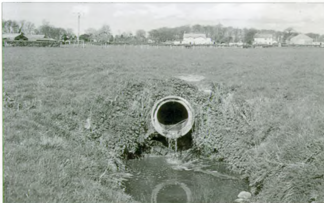
Singleton Village Drain "lack of sewerage facilities".
