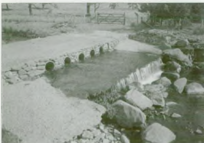
Road Bridge Culverts can cause problems for fish passages.
