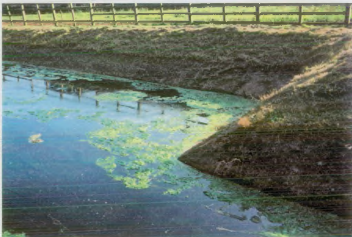
FIGURE 3. CLOSE UP OF ALGAE IN SILT TRAP
