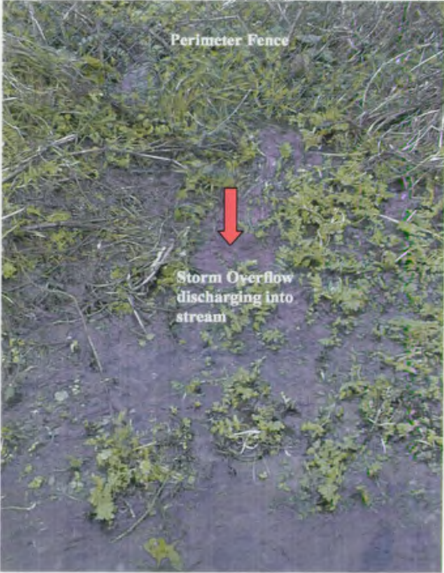
Showing Storm Overflow Discharging under fence into stream
