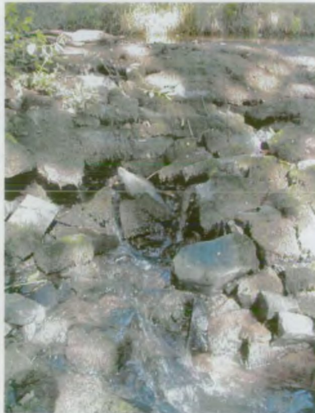
Close up showing breach in weir. During low flow levels all river flow is through breaches not over weir.
