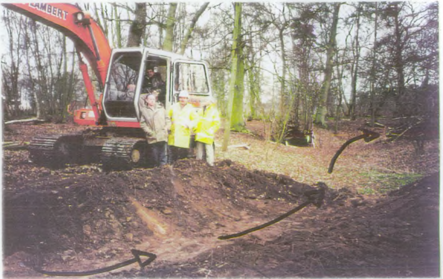
Photo 25 Environment Agency contract staff with the hydraulic excavator used to restore the meandering channel. Arrows show direction of flow.
