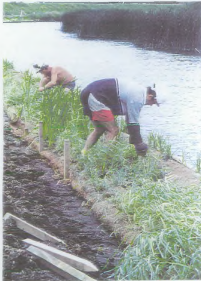
Photo 40 The installation of preplanted fibre rolls and pallets in conjunction with low level piling.
