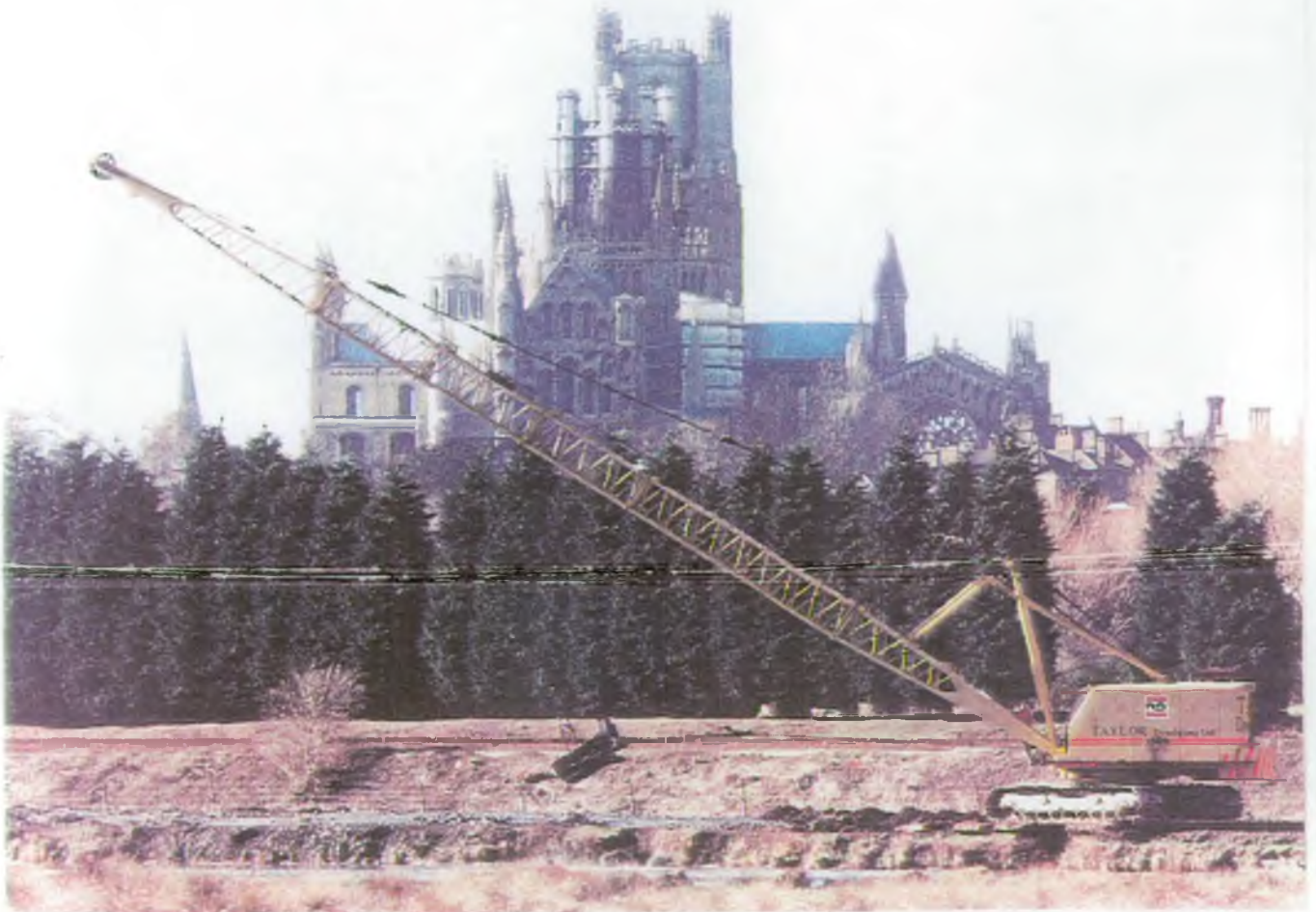
Photo 22 Dredging Works on the Ely Ouse using a dragline with a 70ft reach. Ely Cathedral, widely known as the 'ship of the Fens', is in the background.
