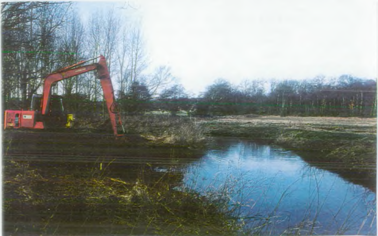
Photo 9 Work begins to reprofile the bank of the Whitewater River at Hoe Rough.
