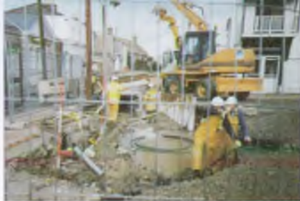
▲ Culvert construction, looking down Beach Lane towards the beach from the town centre
