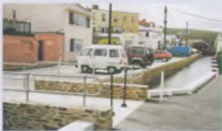
▲ The new culvert now lies beneath where these cars are parked in Beach Lane
