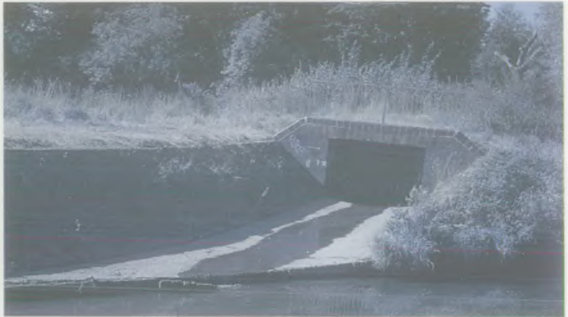
SURFACE WATER DISCHARGE AT BABB'S MILL INTO THE COLE
