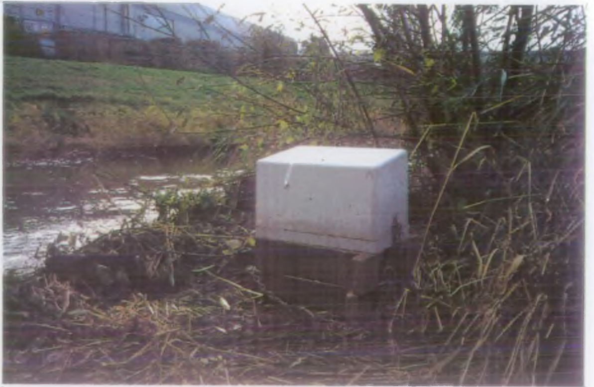
5. MONITORING UNIT AT FIREPOOL SECURED IN GLASS FIBRE BOX
