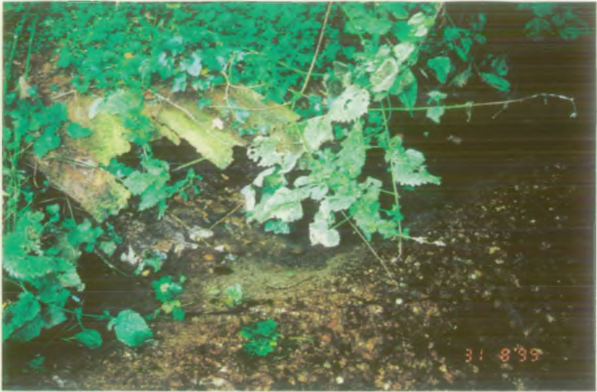
Plate 1. Point of suspected untreated discharge from Chubbs Mill caravan site toilet block.
