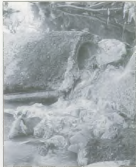
Broken CSO on the River Taff in Pontypridd
