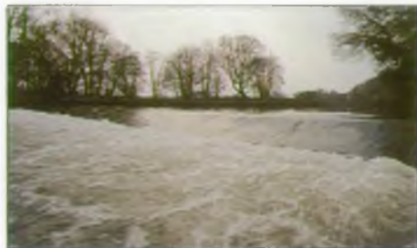
River gauging weir Cored mesur yr afon
