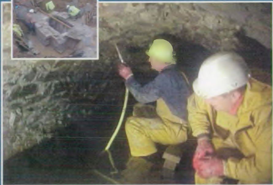
▲ Painting the culvert walls beneath Berrycoombe Road, Bodmin. Inset: Constructing a manhole near Scarlett's Well Road, Bodmin
