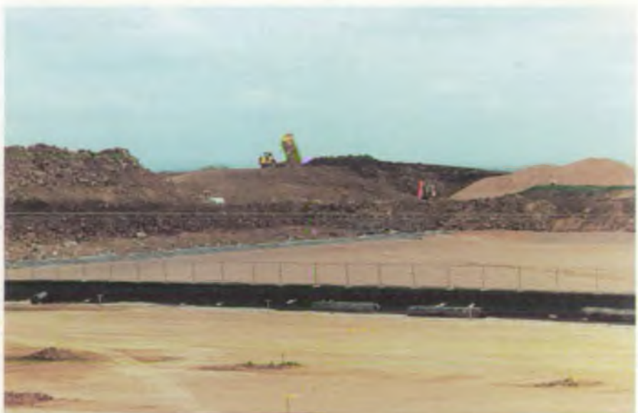
Liner installation at Landfill Site - Landfill sites are no longer simply holes in the ground into which waste material can be tipped. Sites licensed to accept biodegradable waste are now routinely engineered as containment sites using clay or synthetic materials (or a combination of the two) and designed to collect and treat the leachate and landfill gas produced by the decomposition of wastes within the site. North West Waste Regulation Authorities led the country in the development of containment and treatment at landfill sites in their efforts to prevent leachate escaping to contaminate surface or ground water or gas migrating to present a risk of explosion in the vicinity of landfill sites. On many sites, the gas collected is not simply flared-off but used as a fuel to generate electricity and recover some of the energy from the waste.
