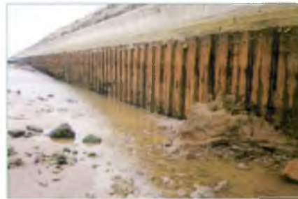
Exposed toe piling to sea wall.
