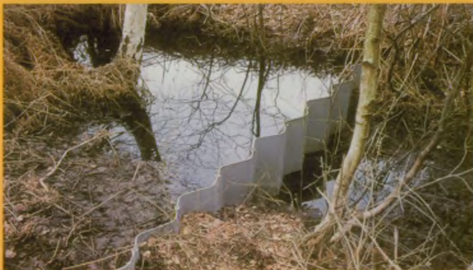
Drainage control installed by English Nature on the Hatfield Moors peat bog restoration area
