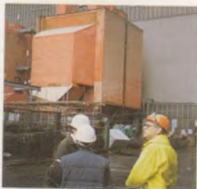
Emissions abatement by electrostatic precipitation at a municipal waste incinerator.
